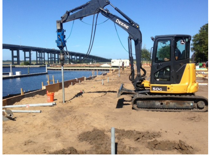
View of installation equipment used to install the helical piles. Equipment consisted of a John Deere 50G Mini-Excavator, an Eskridge 12K Drive Head, and a CHANCE Digital Torque Indicator.
