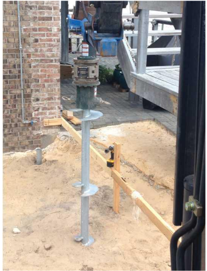
Helical lead section being advanced. Digital Torque Indicator mounted directly above the drive tool.
