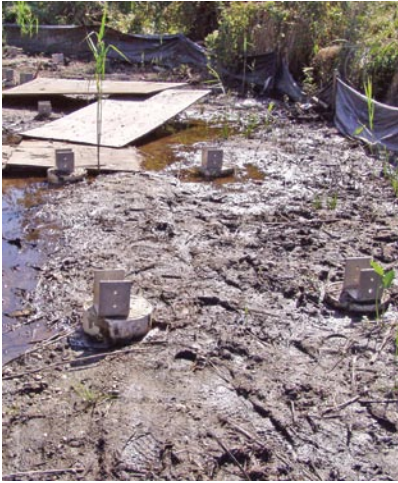
Failed foundation system
