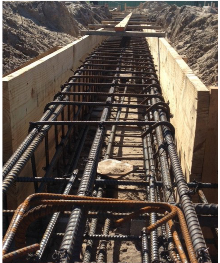
Completed pile system equipped with new construction plate to allow for connection to the new grade beams.
