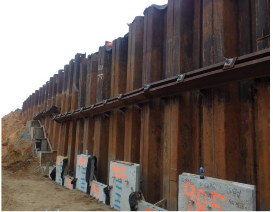
View of the completed anchor and waler system after testing and final lock off.
