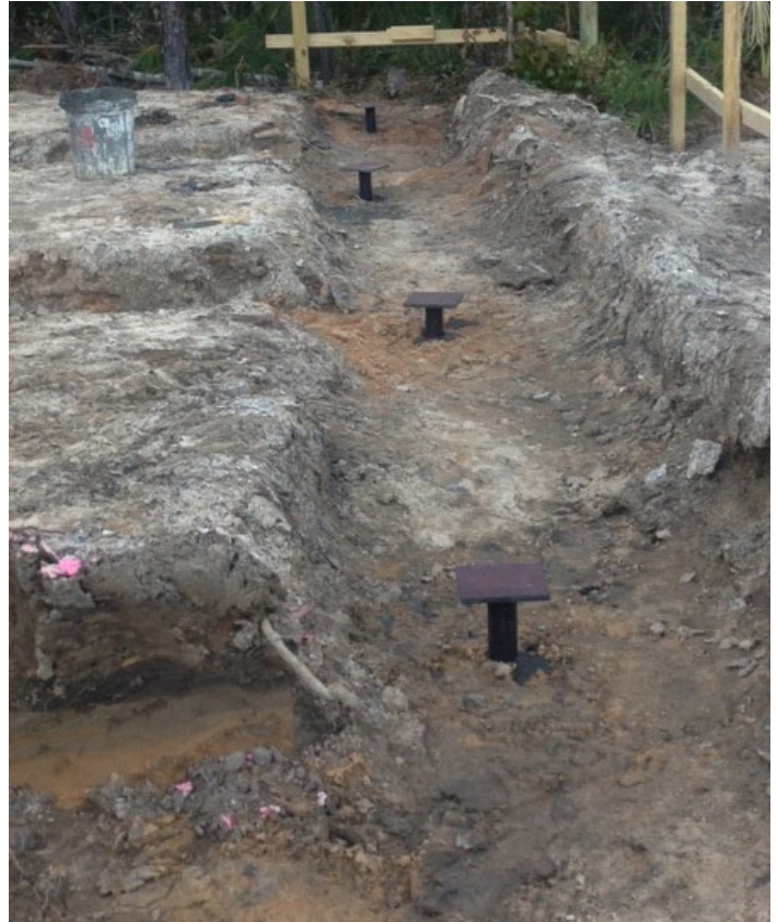
Completed pile system with new construction cap to allow for connection to the concrete grade beams.
